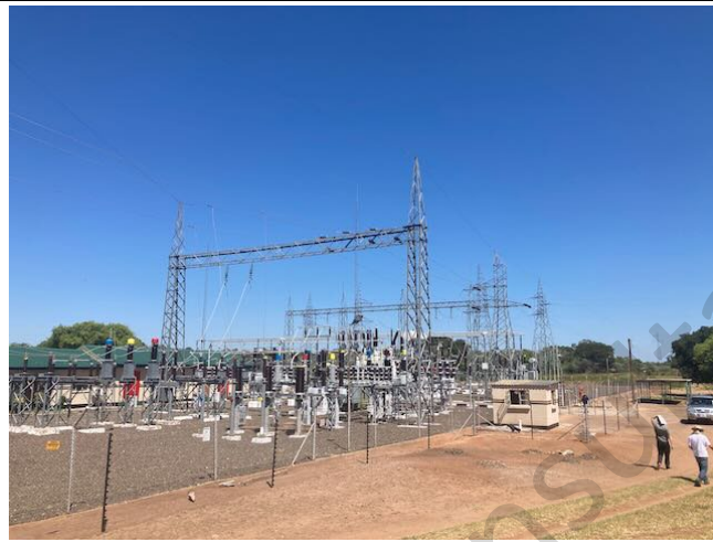
Photo 56: Sesheke substation, where new 220/330kV transmission line from Ngonye Falls will feed into national grid
