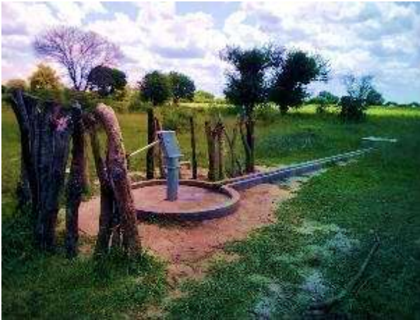
Figure 16: Kandiana Borehole / Handpump
