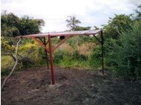
Figure 22: Sikuka Solar Panel and Stand - Muyabalo Community Club
